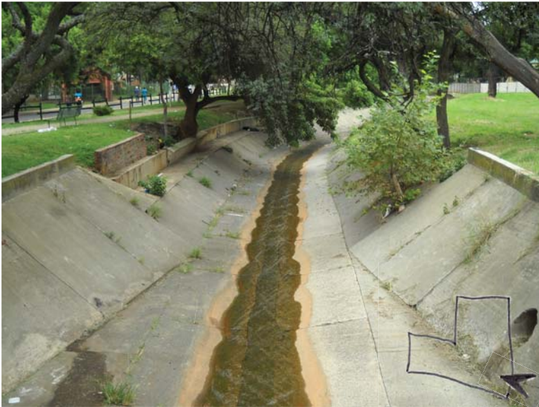
Illus. 5.17: The current concrete channel has a low base flow, but could become a safety hazard during rainstorms (refer to Illus. 5.15 for floodlines). It is not feasible to rehabilitate the channel due to space constraints, but there is an opportunity to clean the water and to beautify the channel. (Author, April 2011)
