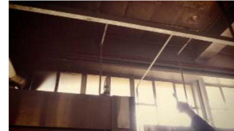
Paraffin and Gas supply pipes
