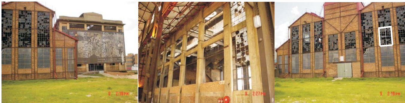
Fig 202. The broken windows of the Turbine Hall.
