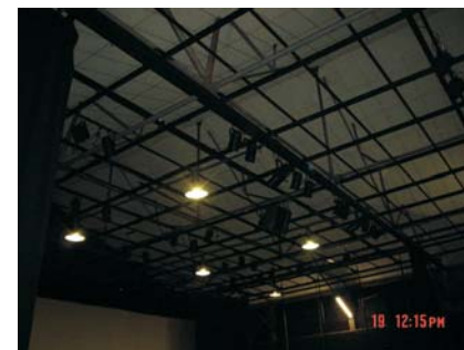
Fig 139. The lighting bridges for stage lighting.
