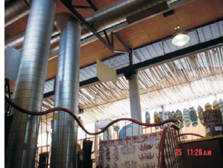
Fig 141. Exposed air conditioning services.
