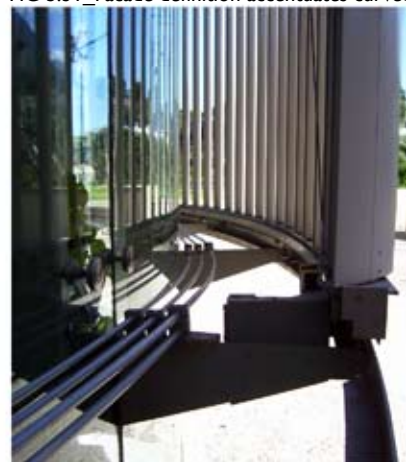
FIG 5.34_Mechanical movement system on facade
