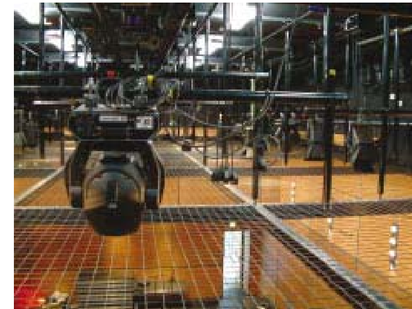
Figure 6.1.6: This system, a 15 x 8m containment Frame, features an integral support structure complete with hangers and lighting grid, and is installed on the first floor of a Georgian villa that is now known as CCA Glasgow. Tension wire grid platforms are woven from stainless or galvanized steel wire rope
