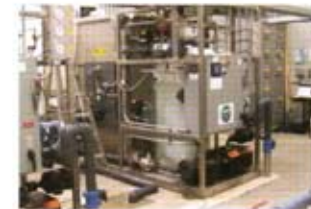
Municipal Drinking Water Township of Toy, OH - 70,000 gpd (263 m 3 /d) Z-BOX M
