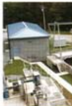
Municipal Wastewater Huntsville, TN - 300,000 gpd Packaged Equipment Skid
