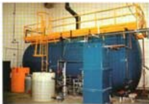
Decentralized Treatment Office Park, Oakville, ON - 17,500 gpd (66 m 3 /d) ADF* 2-MOD S
