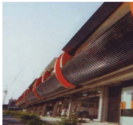
116. State Emergency Services Headquarters - Fractured Facade
