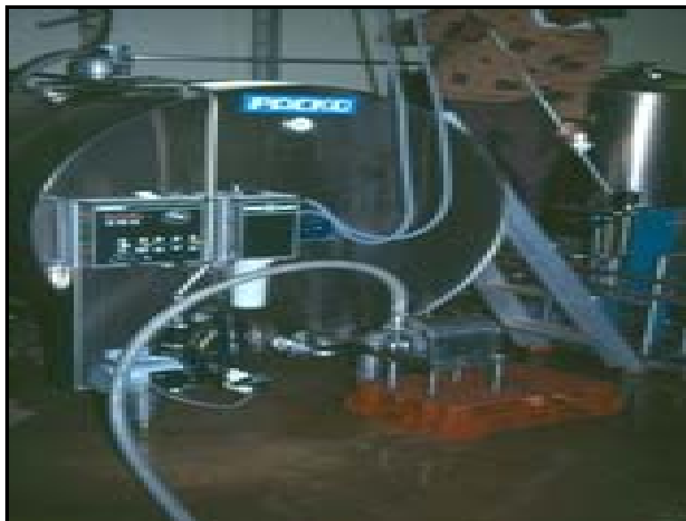
Plate 2. 10: Electronic monitoring and cooling system on bulk tank
