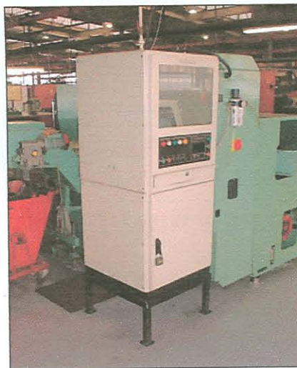
Figure 5.18: Steel enclosure for monitoring electronics
