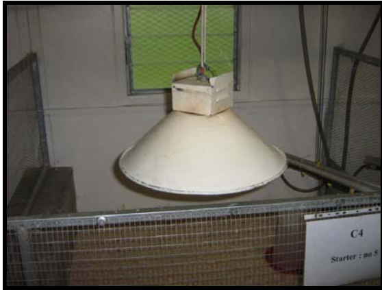
Figure 5.3. Heater hanging from the roof
