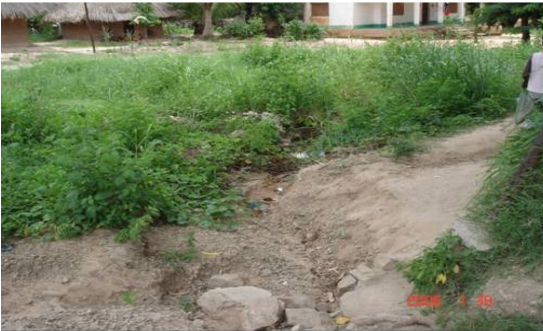
Picture 4: shows traditional technique used by rural Community to prevent growth of soil erosion.
