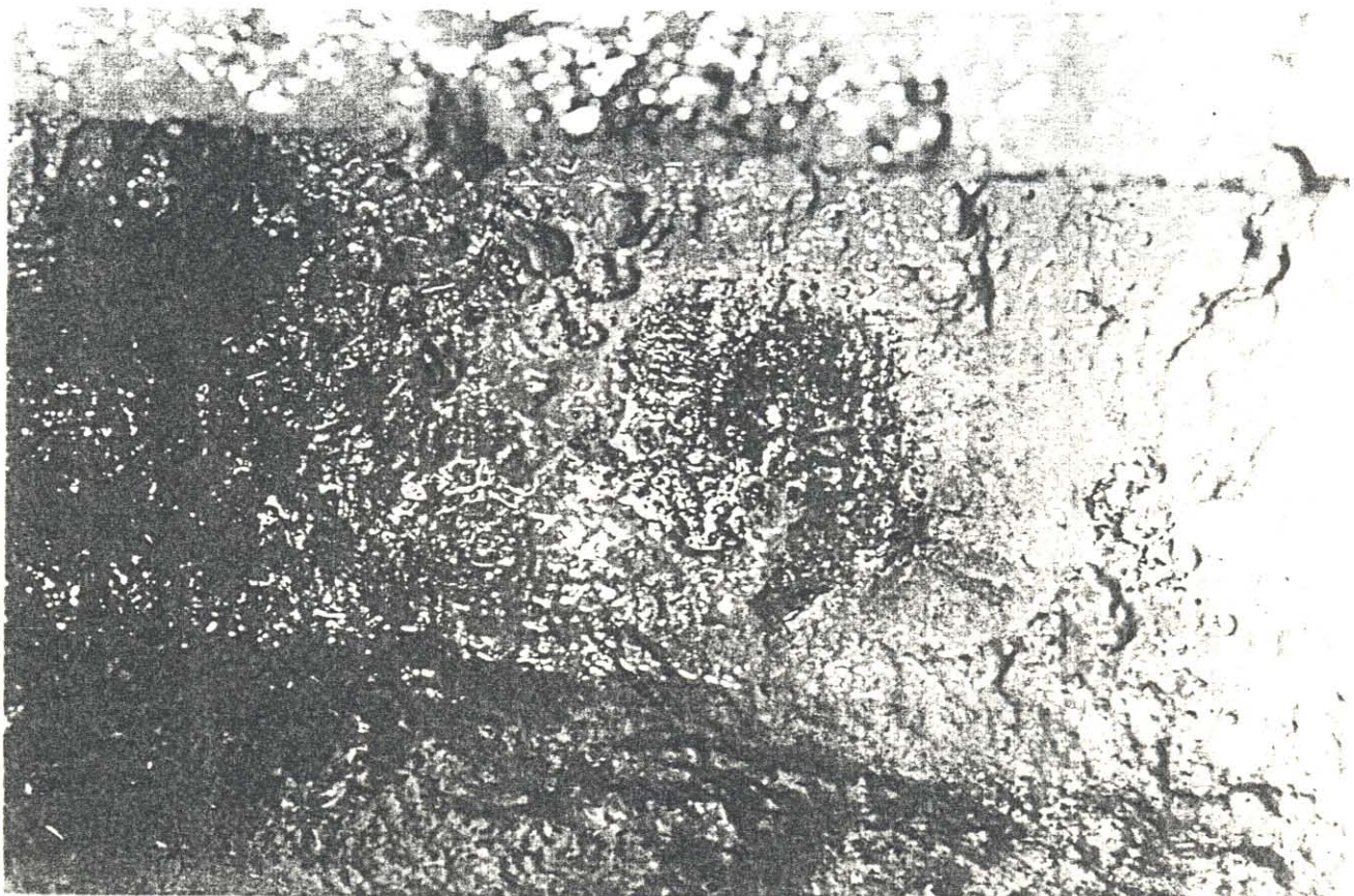
Figure 4.9 : Strainer box at Grootvlei Power Station after three weeks of biodispersant/biocide treatment showing softened nodules on surface (A) and loss of black colouration in underlying pits (B).
