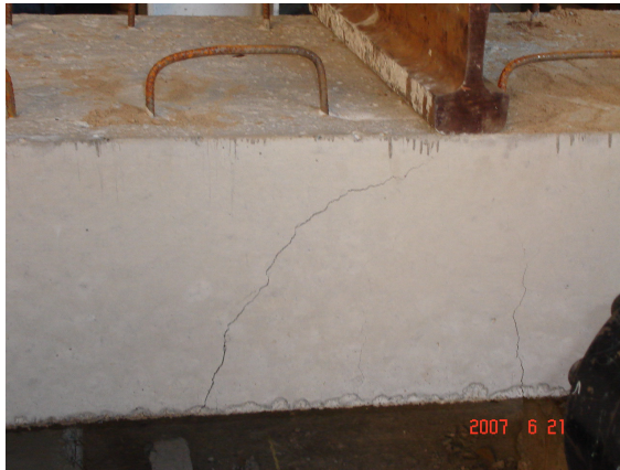
Solid slab crack
