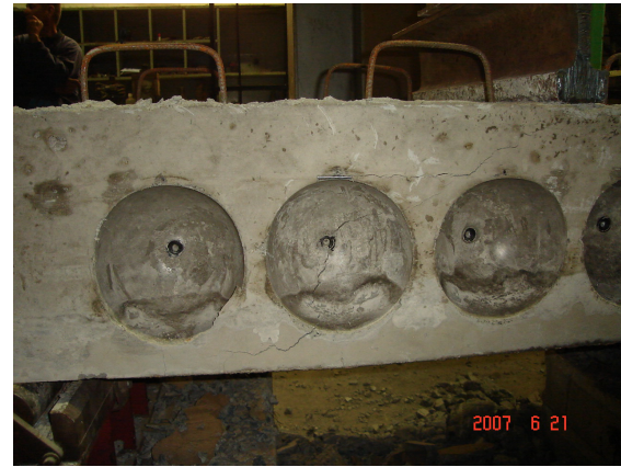
Cobiax slab crack
