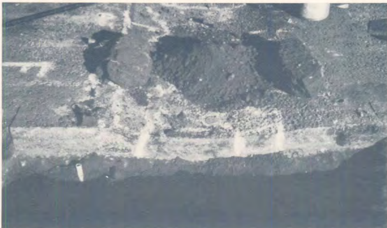
(c) Recovered granulated upper subbase material within the trafficked area. Note blocks of the same material recovered from the untrafficked area.
