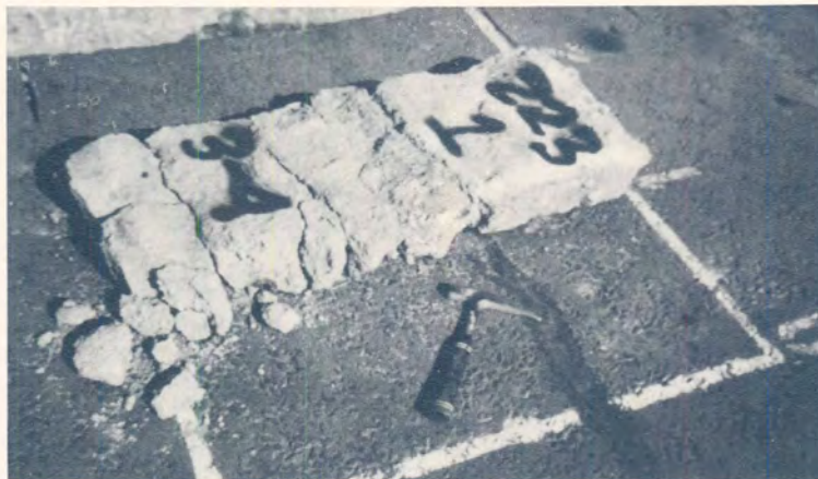
(b) Recovered upper subbase after 20,6 ME80s. (Semi-saturated). Note the position of the longitudinal crack. The other cracks are traffic associated. (Measuring points 3 to 4).
