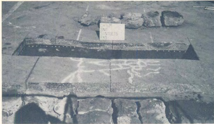
(a) Cross profile across the test Section 1. Note the heaving of the asphalt as a result of the erosion action inside the trafficked area during the EPWP state.
