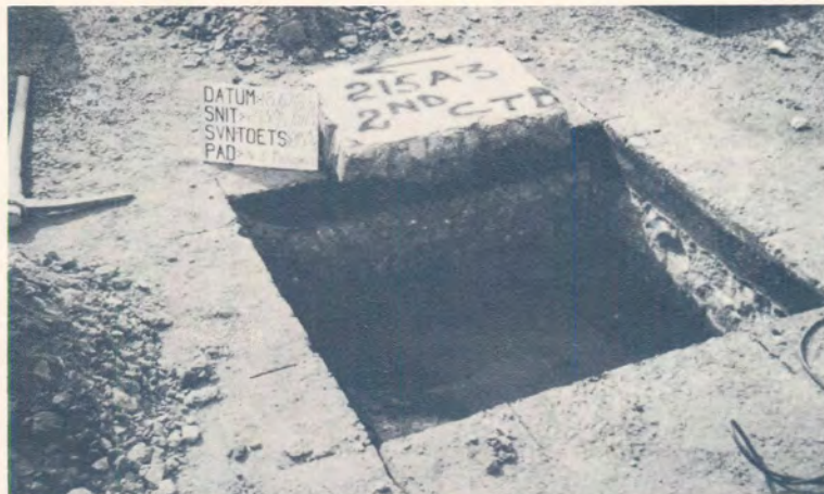
(b) Successful recovery of a solid block of stabilized material from the lower stabilized subbase layer. Note smooth interfaces between the layers.
