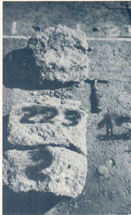
(b) Recovered lower subbase layer after 20,6 ME80s on SECTION 1 (saturated) at measuring points 11 to 12.
