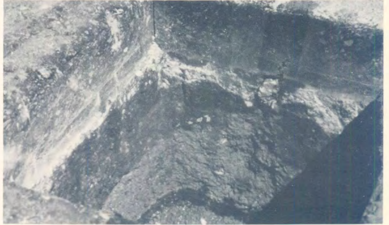
(b) Relative low pH zone at the position of the crack (dark red colour – high pH zone), determined with Phenolphthalein.
