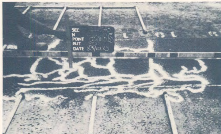
(c) Maximum rut of 80 mm on MDD12. Note the fatigue cracking of the asphalt layer. E80s on wet test section: 6,8 \times 10^6
