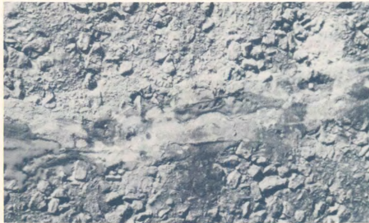
(b) Fines starting to pump through the longitudinal crack.
