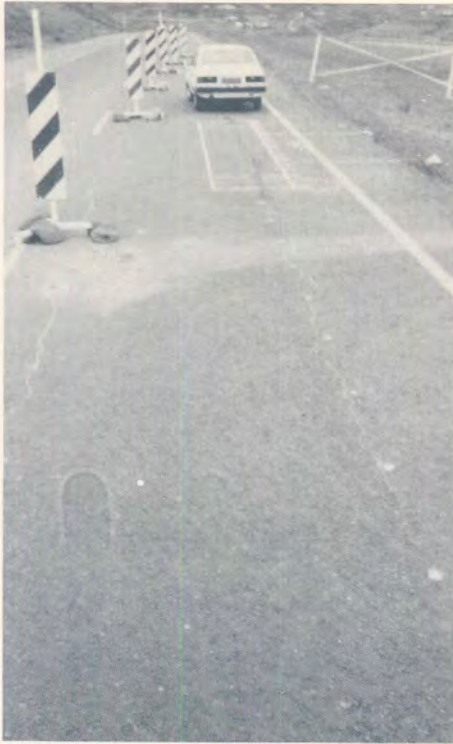
(a) View of HVS site on the fast lane of the south bound carriageway. Note the settlement cracks.
