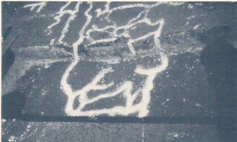
(b) Visible cracks on top of the upper stabilized subbase layer after the removal of the asphalt in (a).
