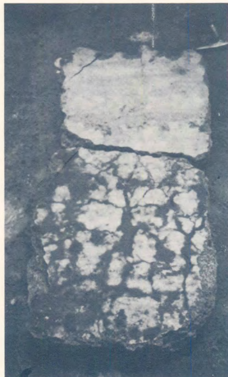
(b) Recovered cracked upper stabilized subbase layer after 3,6 \times 10^6 E80s.
