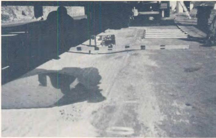
(a) Surface condition of Section 1 after the EPWP state, (62 mm rut after 2067 repetitions at (100kN) Note the white water inlet pipes both sides of the Section.
