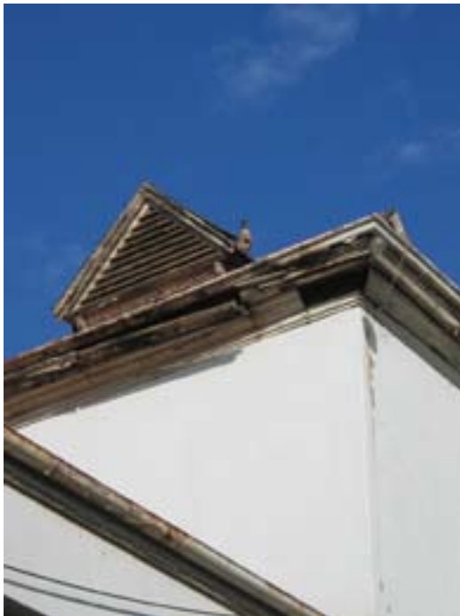
Image 16: Roof vents are placed on all roofs of the building
