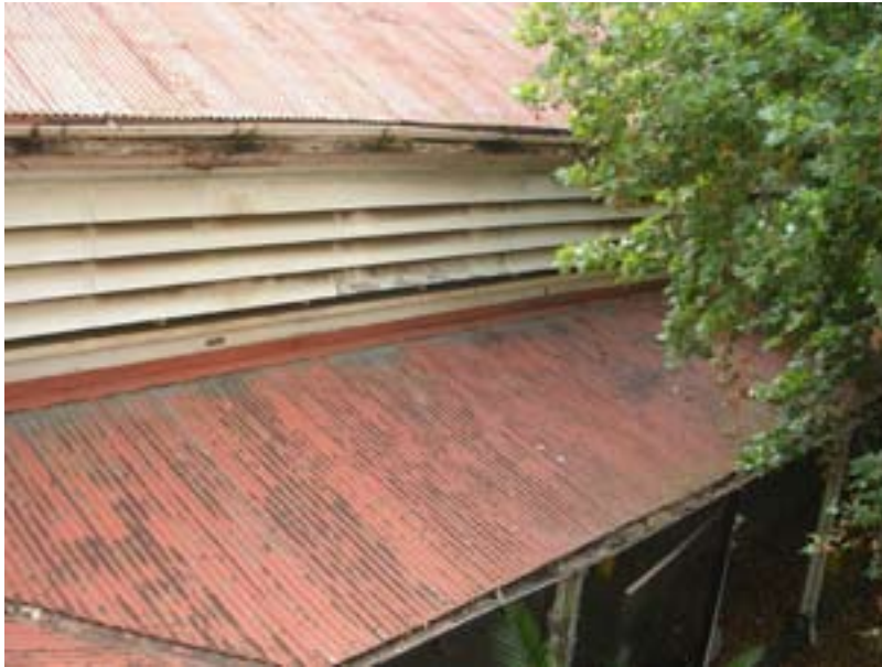
Image 38: Louvres were later added in front of all clerestory windows of the east and west wing
