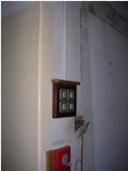
Image 40: Evidence of later added electricity is found throughout the building
