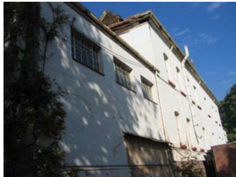
Image 29: Three later added steel windows can be found on either end of the northern wing
