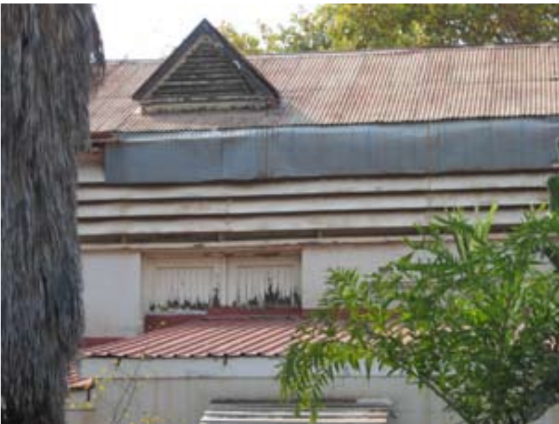
Image 8: The roof of the late addition stretches right across the 'wagon doors', blocking them
