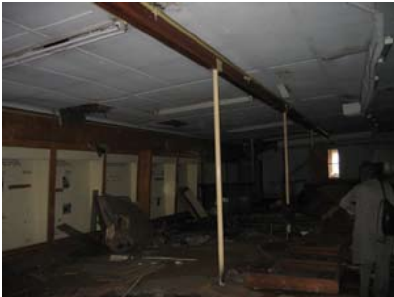
Image 48: The interior courtyard addition is left damaged by water and lack of maintenance
