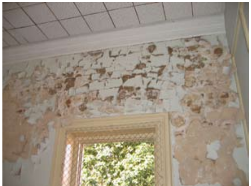
Image 17: The PVA paint layer is peeling off the lime-based paint. (This photo was taken in the northern upper wing, but also applies to the 'tower' first floor.)
