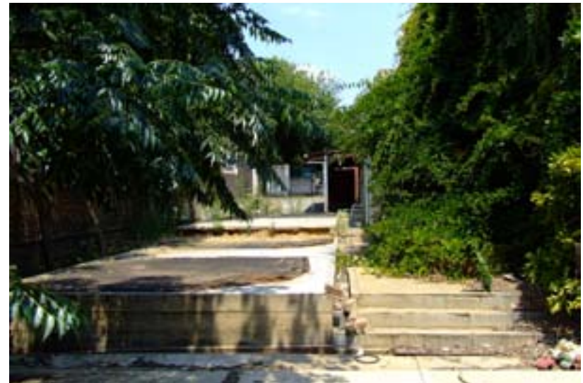
Image 9: Uneven blocks protrude from the ground level on the eastern side of the building
