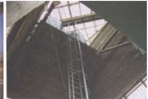
Figure 56: Water tanks in tower
