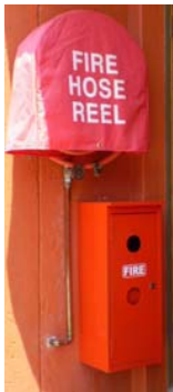
Figure 6.8.3.1 Fire fighting equipment
