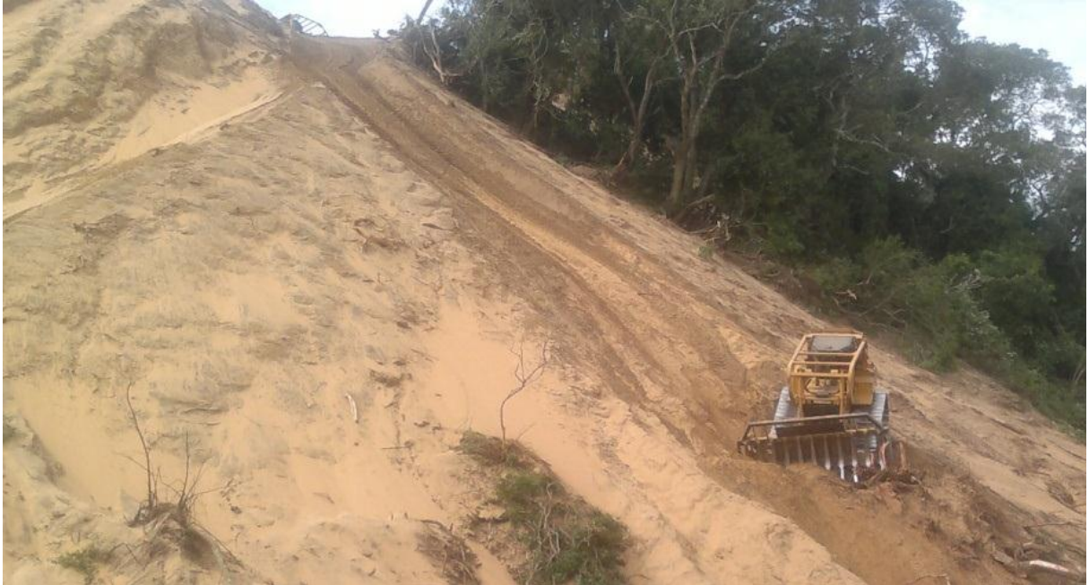
Plate 1. Heavy machinery is used to clear vegetation from the coastal dunes prior to the extraction minerals from the sand.
