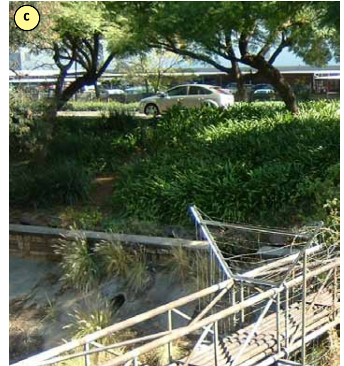
FIGURE 40. VIEW SOUTHWESTWARDS FROM THE PROES STREET BRIDGE - THE LEVEL DIFFERENCE FROM THE PROES STREET INTERSECTION TOWARDS THE CHANNEL DROPS BY MORE THAN 2.5M.
