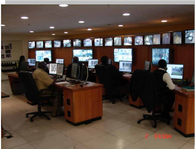
Figure 10: Security control room
