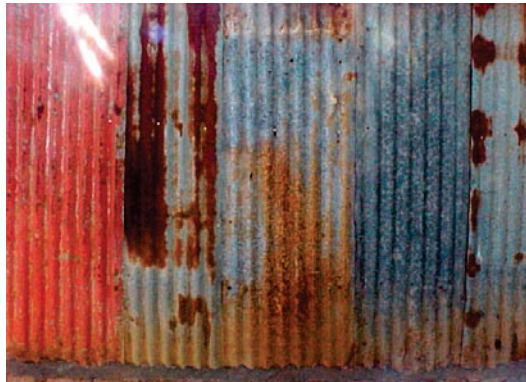
Figure 4.11 Second-hand profiled steel sheeting is used to build houses in both informal and formal settlements. The untreated material ages over time due to harsh climatic conditions, leaving it stained. The dialogue of this material is to be continued on the skin cladding system of the overnight accommodation building
