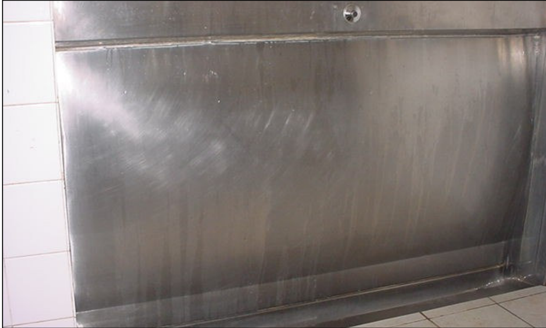
Figure 26: Modified urinal flushing mechanism
