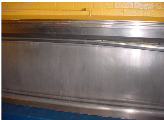
Damage to urinal
