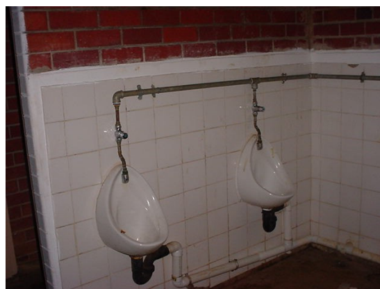
Drainage plumbing makes cleaning difficult
