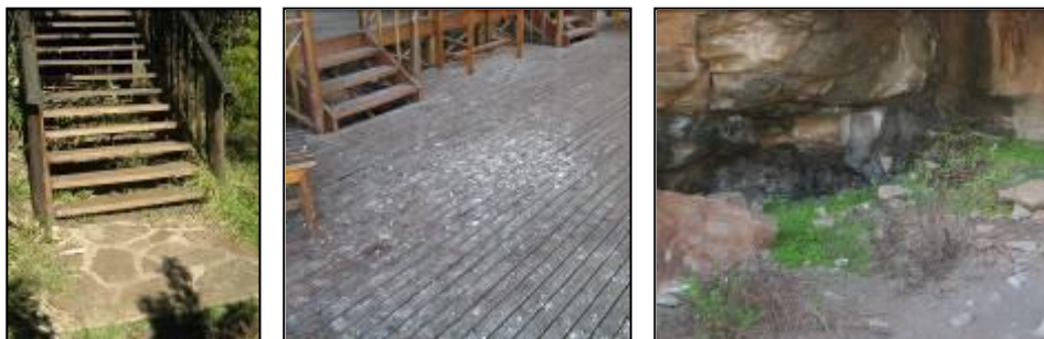
Figure 7.30: Left: The new stairs replaced after a fire at the second overhang. Middle: Bird faeces. Right: Vegetation growth near the rock surface at Main Caves (Photographs: C.L. Fordred).
