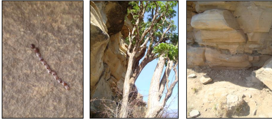
Figure 7.6: Examples - of the natural weathering elements – insects ( left ), shade ( middle ) and dust that contribute to the deterioration of the rock surfaces at Sigubudu Shelter ( right ) (Photographs: C.L. Fordred).
