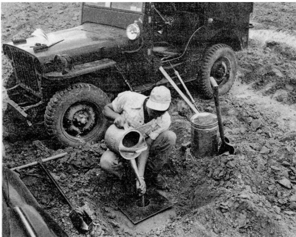
Figure 1.2: Determining density by replacement with sand of known density (After Design of small dams, 1965).
