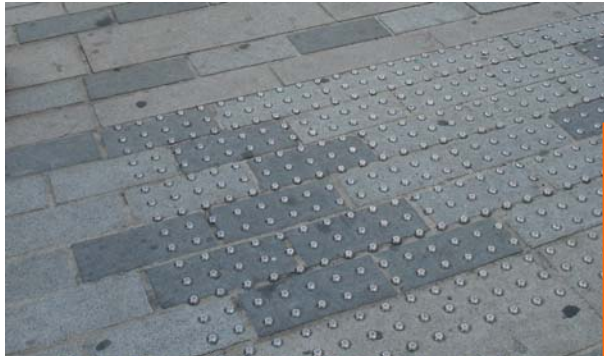
fig.6.45: Anti slip studs in pavement
