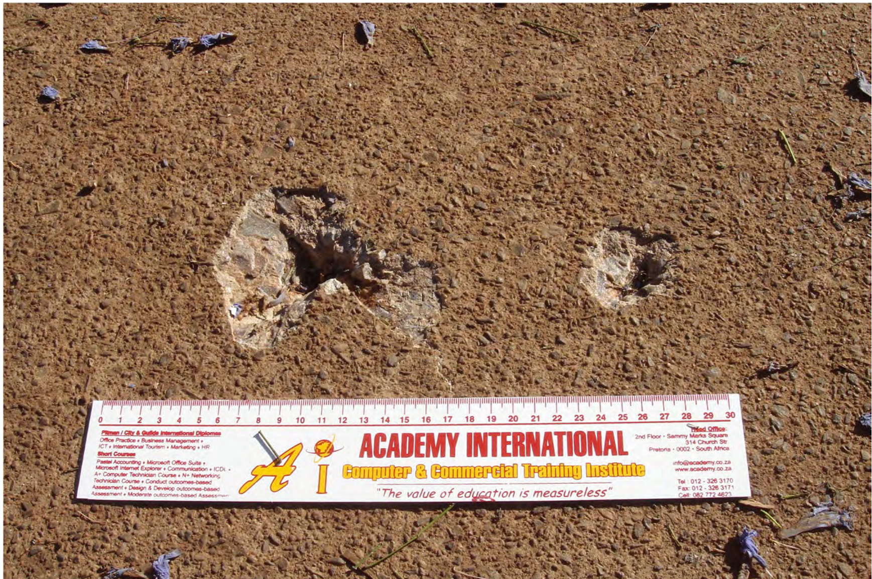
FIGURE 3. Photograph of the crater on the pavement.
