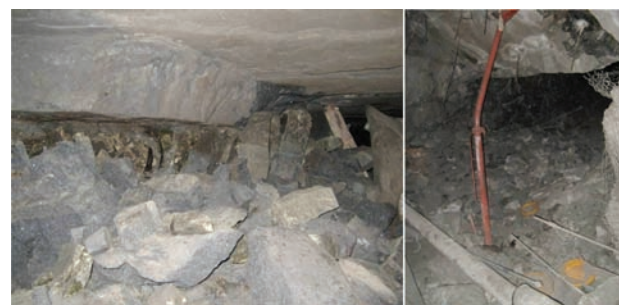
Figure 17—Interest mode of pillar failure at Mine B. For this pillar, a clay layer was found between the upper LG6A chrome and the pyroxenite below it. This slippery layer facilitates the fracturing of pyroxenite, causing it to scale out (left). The failures led to large amounts of convergence as can be seen in the photograph on the right
