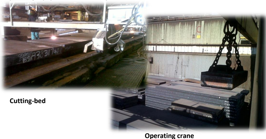
Figure 9 : Operating equipment in the slab yard
