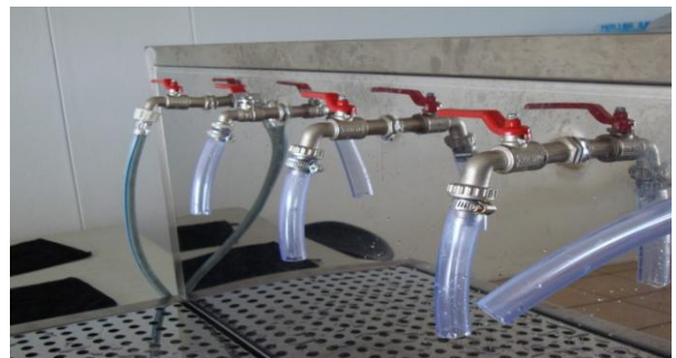
Figure 3. Valves used to fill bottles.
