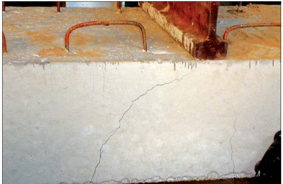
Photo 2 Observed crack patterns at failure for the solid samples (UP 2007)
