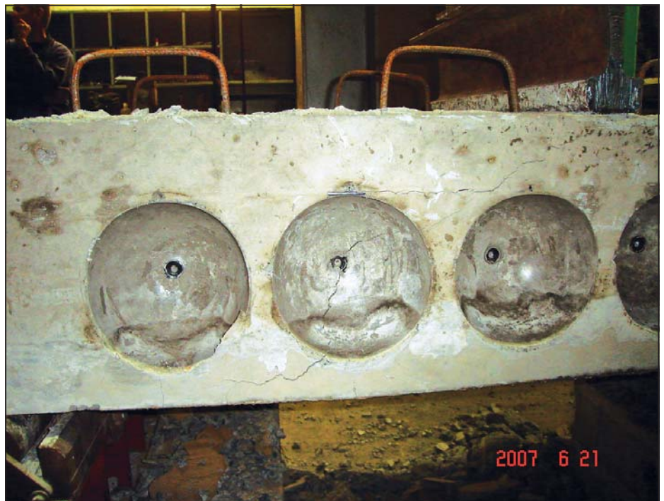
Photo 3 Observed crack patterns at failure for the SVF samples (UP 2007)
