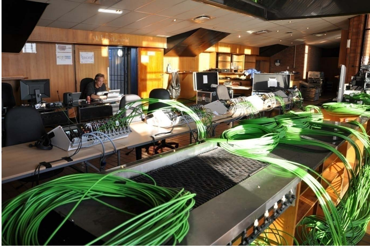
Figure 26: Cabling for CCR layout 2
