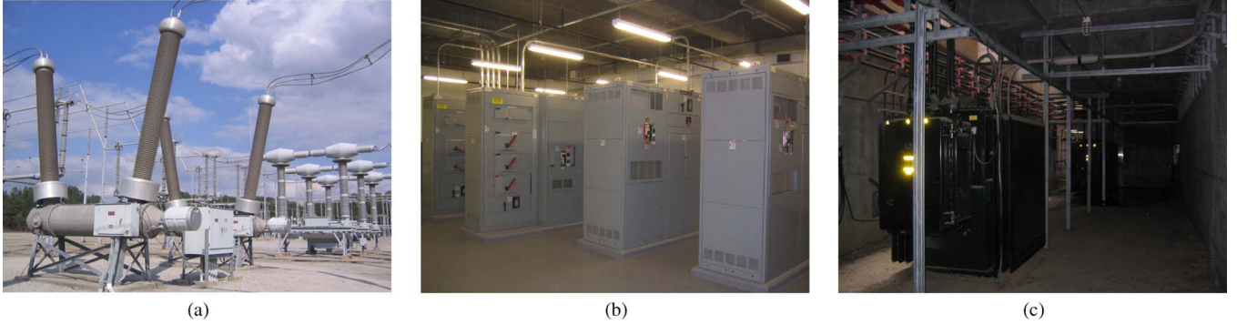
Fig. 1. Experimental sites. (a) Outdoor 500-kV substation environment, (b) indoor main power room, and (c) underground network transformer vault environments.
