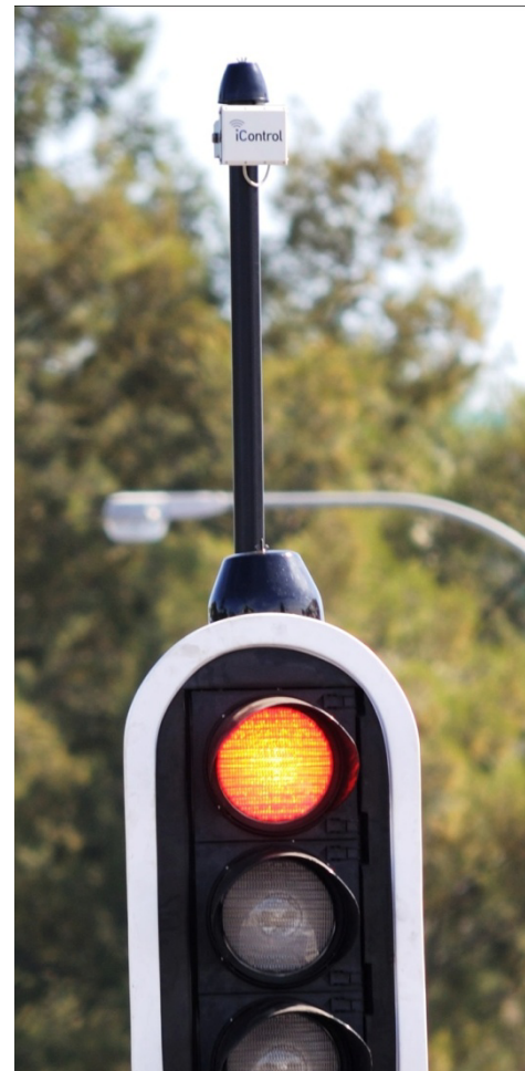
Figure 1: Scanning radar installed in Malmesbury
