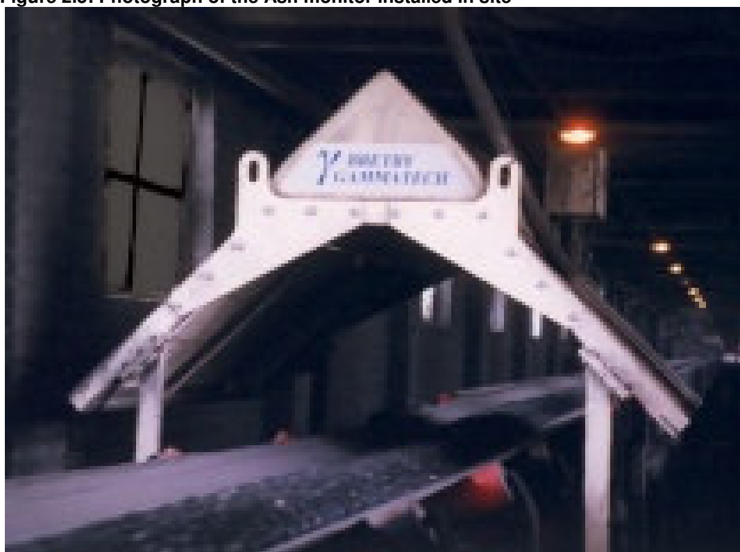
Figure 2.5: Photograph of the Ash monitor installed in site
