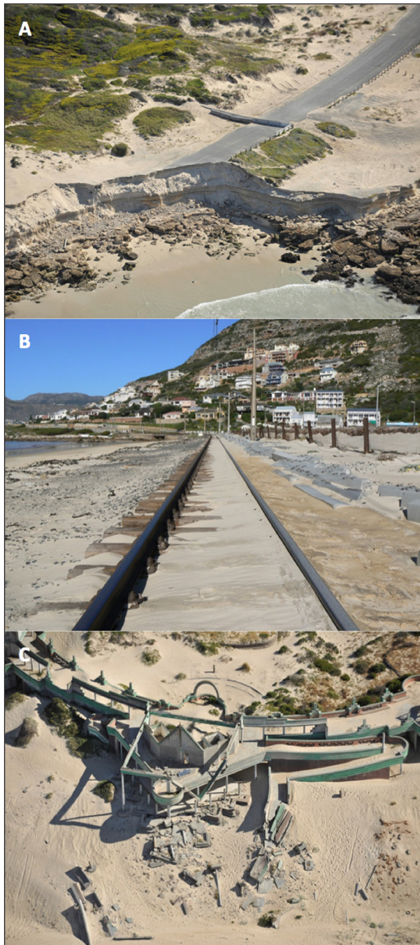
Figure 17: Examples of the coastal vulnerability of False Bay. Exposure of (A) infrastructure to erosion at Monwabisi, (B) the railway to erosion and wind-blown sand at Glencairn, and (C) broken infrastructure at the Macassar Beach coastal public resort creating an unsightly and unsafe environment (photo credits: B. Sutherland and D. Colenbrander). DOI: https://doi.org/10.1525/elementa.367.f17
