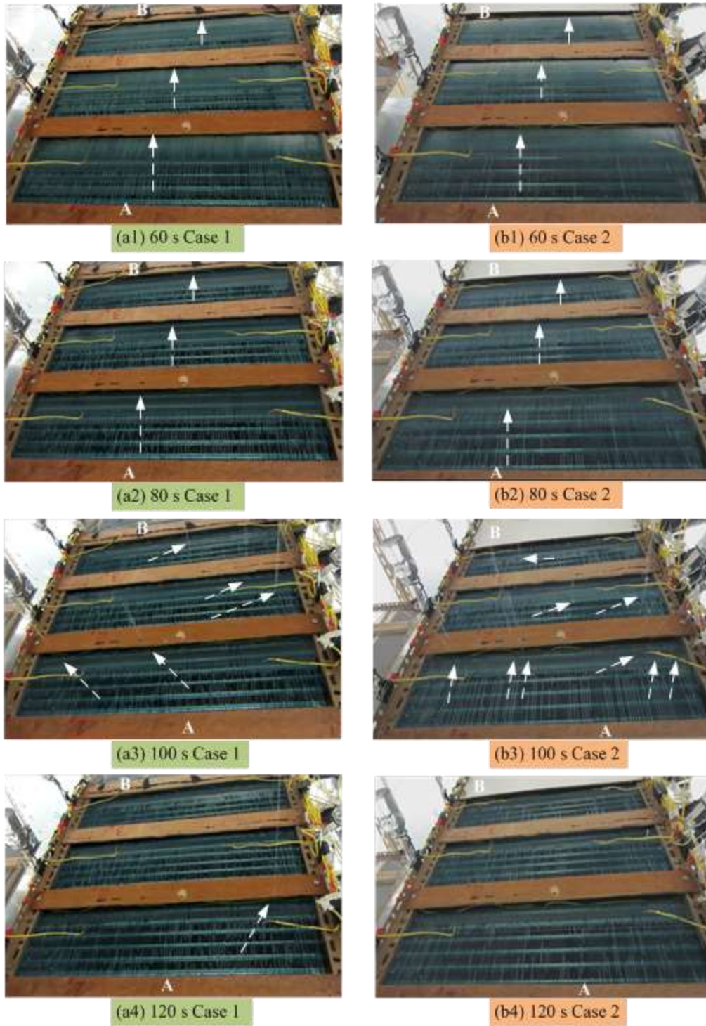
Fig. 9 Airside surface conditions of the outdoor coil during defrosting in Case 2 and Case 3 (eight photographs)
