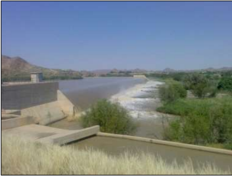
Figure 24: Typical measuring structure/weir (Neusberg, SA)
