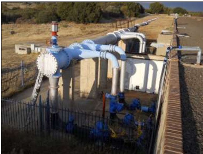
Figure 22: A photo of a pressure reducing station at the Brandkop Reservoir, SA
