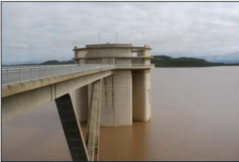
Figure 23: A photo of the intake to the Orange-Fish Water Transfer Scheme, SA
