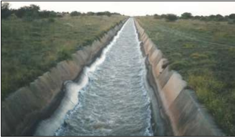
Figure 18: Example of a concrete lined chute at Schoenmakers in the Orange Fish WTS
