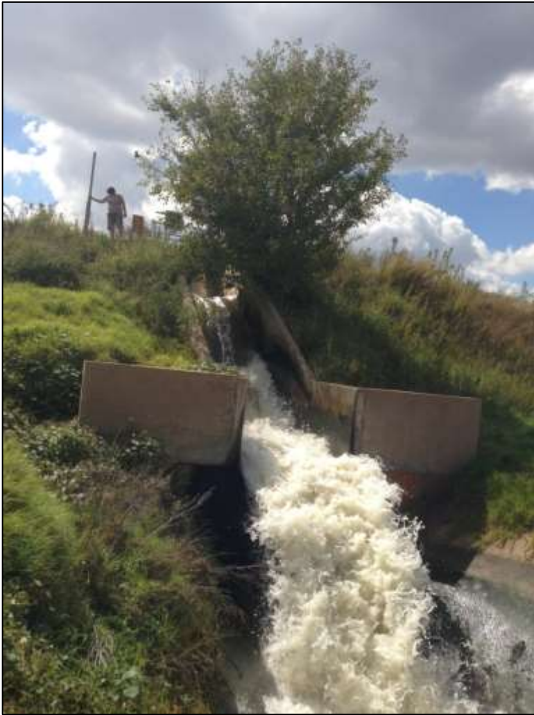
Figure 25: Rooiwal Wastewater Treatment Works outlet
