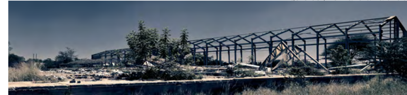
Figure 03 | 49. Main steel portal frame
