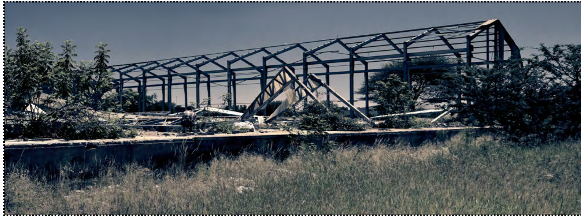
Figure 03 | 34. Main steel portal frame
