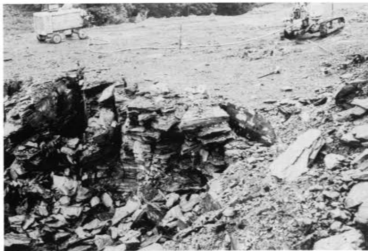
Plate 7: Drilling and blasting of road cutting between Boston and Merrivale in Natal (Sampling point for M1)
