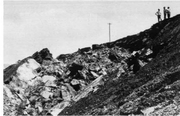
Plate 6: Slip of large volume of material on inclined bedding plane in road cutting at Peter Road, outer ring road, Durban (Photo: D. Weston)
