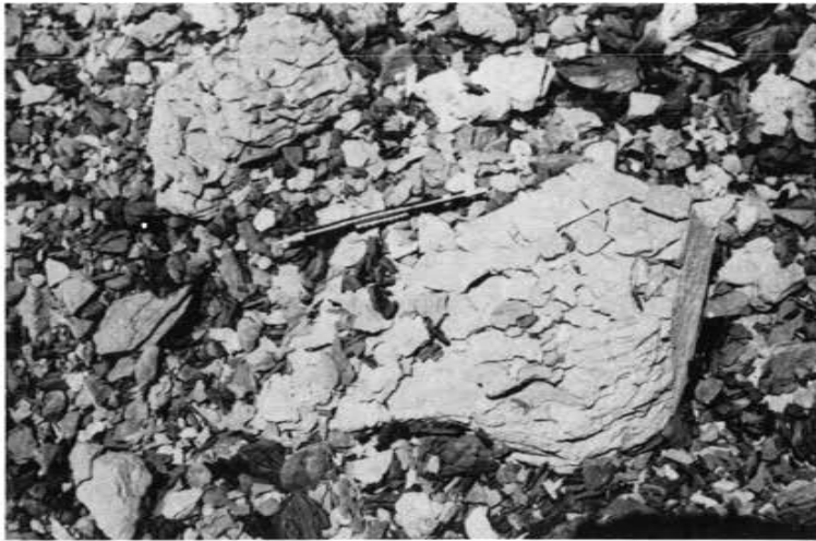
Plate 1: Disintegration of Ecca shale at Peter Road cutting on outer ring road, Durban
