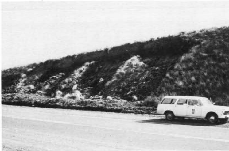
Plate 5: Slips of vegetation and topsoil on slope between Ficksburg and Fouriesburg
