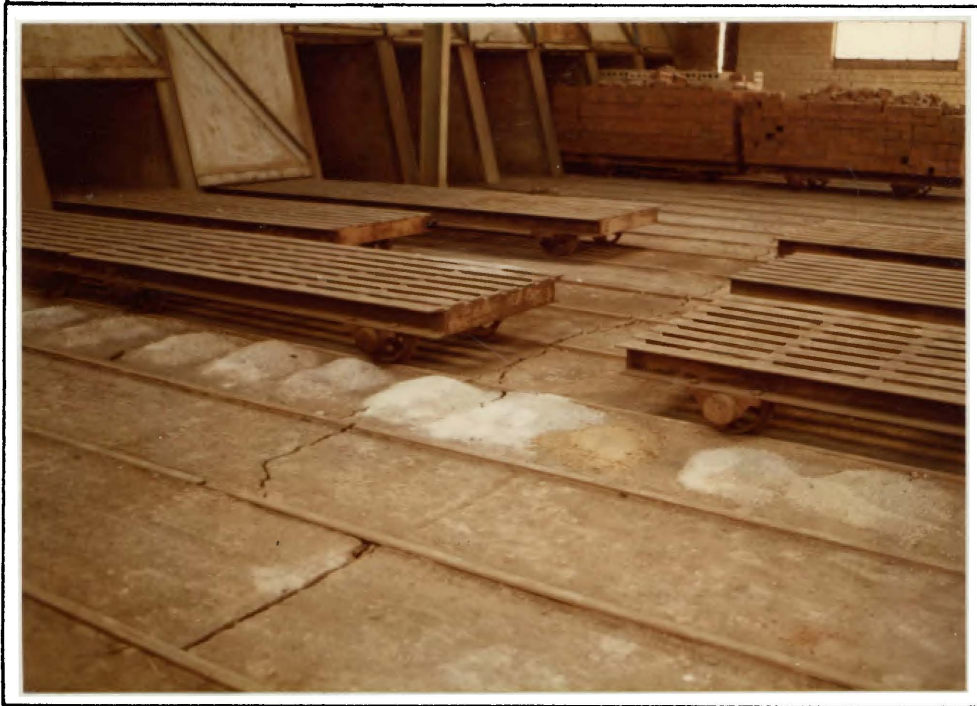
Showing cracking along floor of the Down - draught dryers at Driefontein Brickworks caused by differential subsidence.
