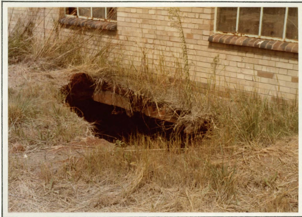
The 5m diameter Sinkhole (Sinkhole 17) which occurred at Driefontein Brickworks on 18 th February, 1980.
