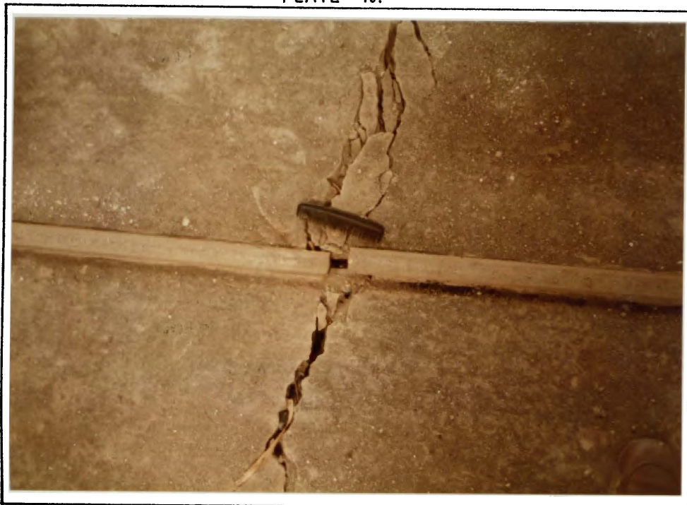
Detail of cracking along floor of the Down - draught dryers at Driefontein Brickworks caused by differential subsidence. Note the dislocation of the rail.
