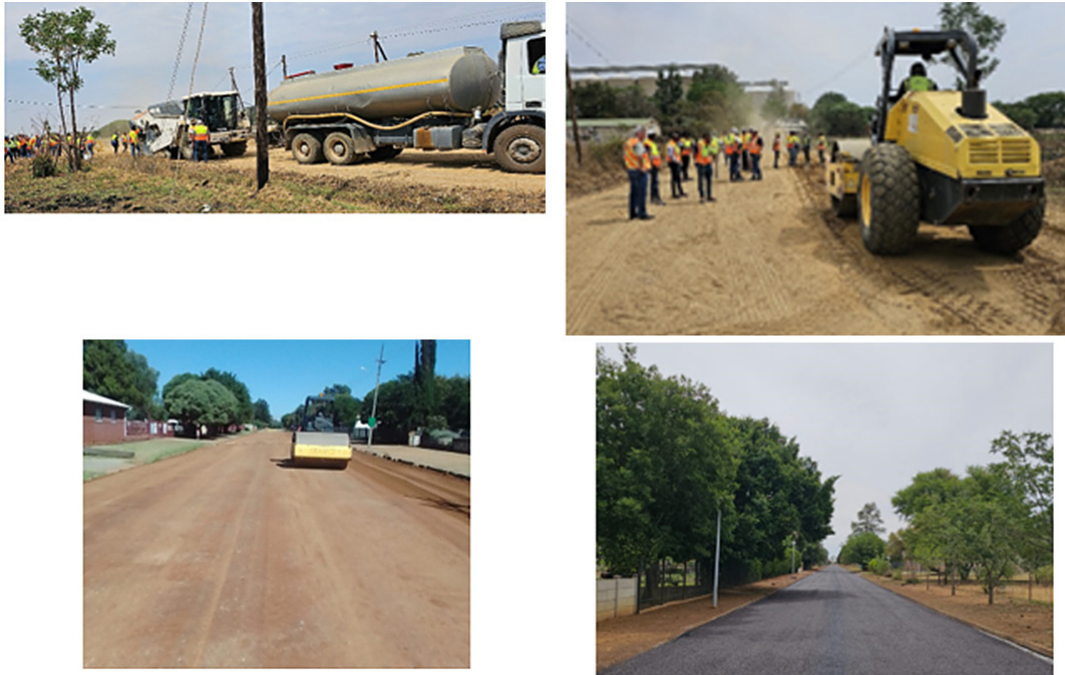
Figure 7: Images Clockwise. West street linking to silos Leeudoringstad, compaction behind recycler, completed Botha street with slurry finish
