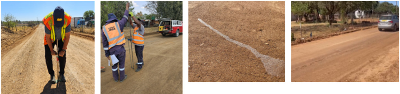
Figure 10: Illustration of alternative testing. RCCD testing, DCP testing, water resistance testing bottom with top dust absence behind travelling car and experimentation with tack coat types and application
