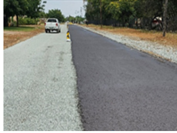
Figure 9(b) Vrede street chip and spray followed by slurry application in process
