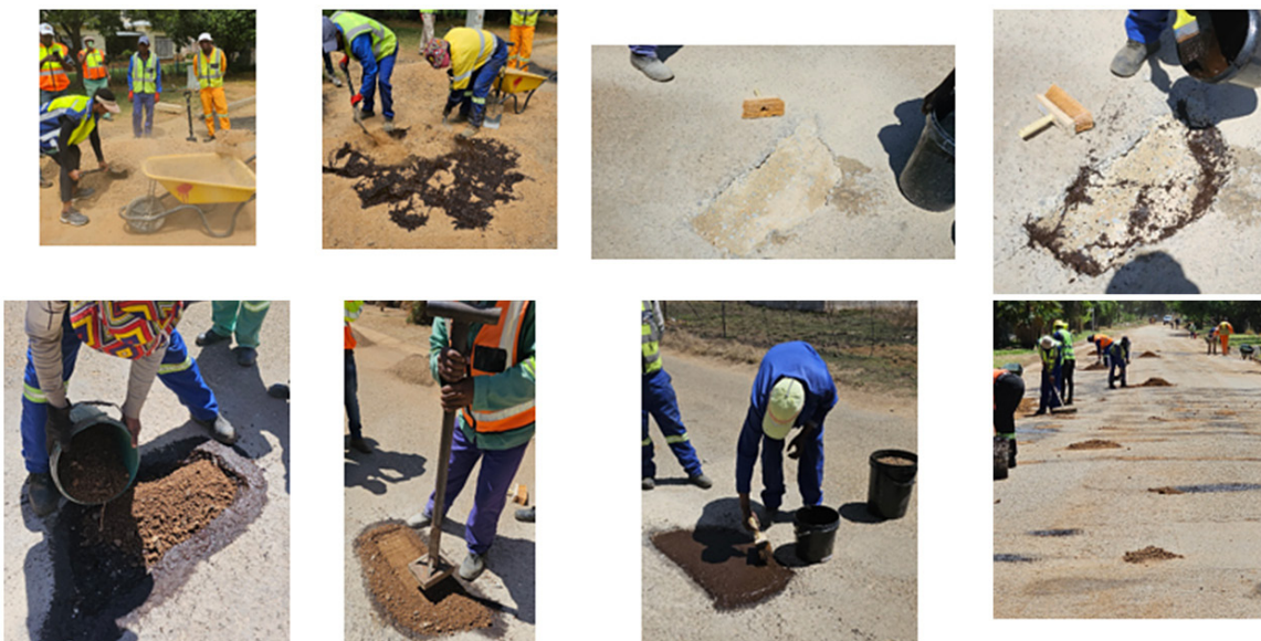
Figure 6: Clockwise, Ease of hand mixing G5 and NME demonstrated, pothole cleared of all loose material, sides and bottom painted with NME, mixed G5 with NME placed in pothole with lips also painted with NME, compacted with tamper, NME painting on top after compaction and large scale production with local labour on Smit Street, Wolmaransstad
