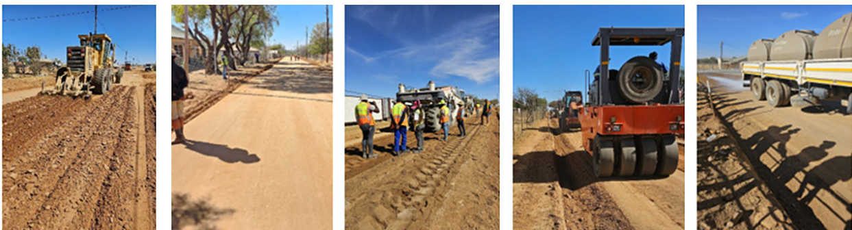
Figure 4: Witpoort gravel preserved street: Grader preparation before hand, compaction before recycling, recycler trainn mixing in 75mm thickness NME, compaction with heavy vibratory roller and pneumatic, Clearspray with water cart
