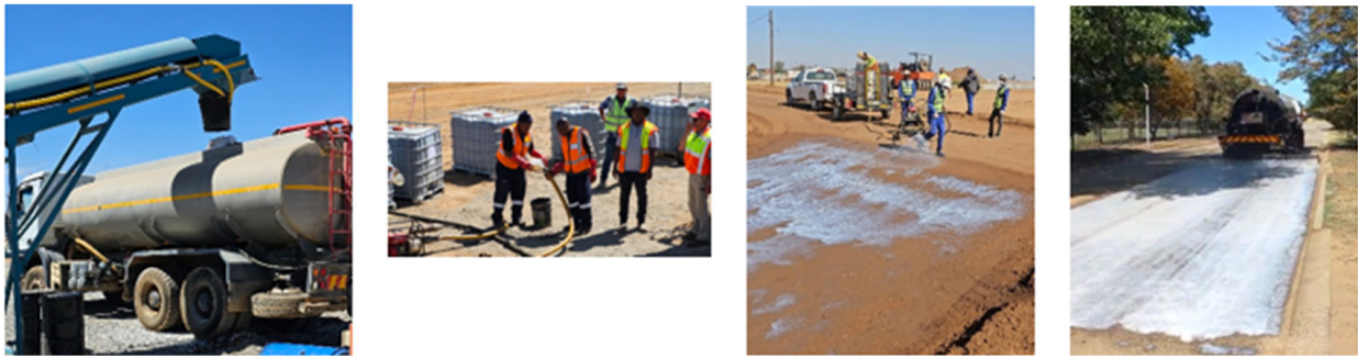
Figure 5: Precise water volume measurement in water cart, NME addition from Flowbins, Clearseal application by hand spray, Clearseal accurate spray by spreader and tack coat on prepared surface
