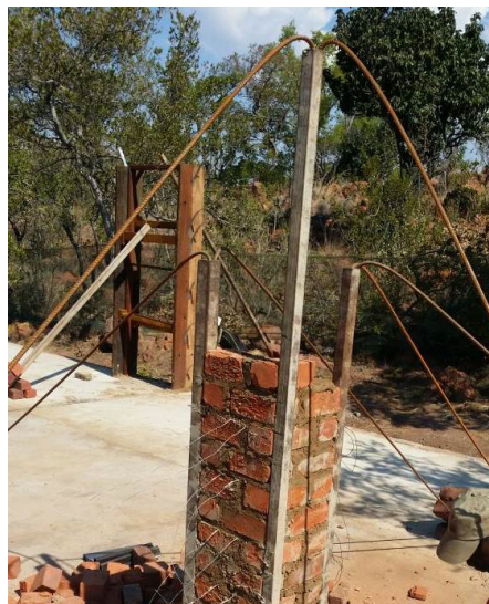
Figure 6: Brick pillars with brick force shown as variation for end stops as well as door with sleeper planks around door frame before shutter work erection
