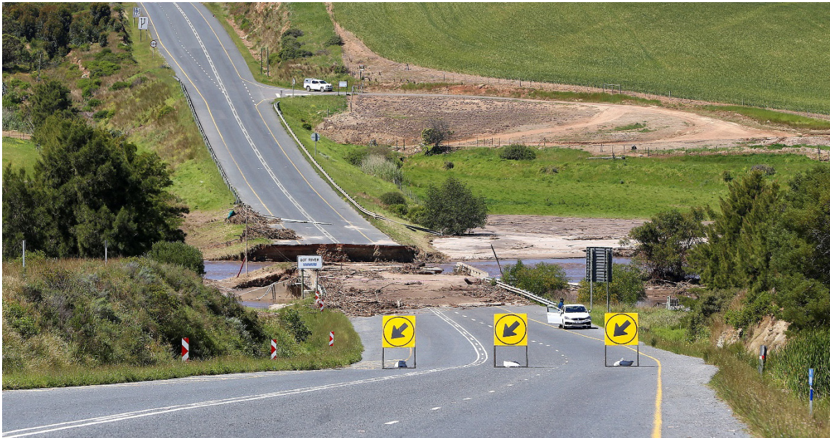
Figure 1: Damage to the N2 at Bot River (photo courtesy of Independent Media)
