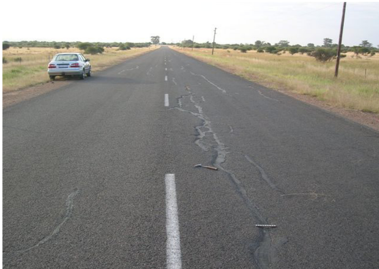
Figure 2: Longitudinal cracking on road P65/1 near km 9 after three years in April 2009
