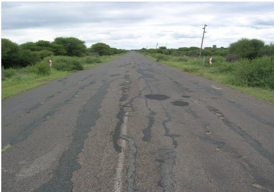
Figure 3: Condition of P65/1 near km 9 in February 2024 (this culvert had been reinstated due to settlement during construction)
