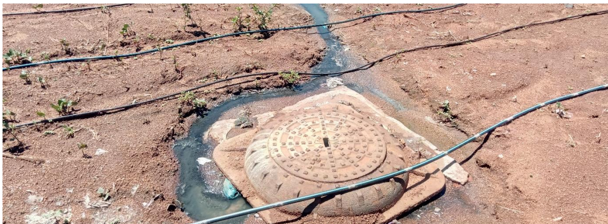
Figure 3-2: Leaking sewage line at the Rooiwal Agri-park on 2019-01-09
