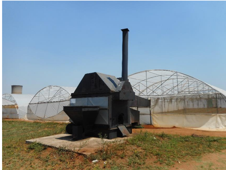
Figure 2-4 : Dysfunctional tunnel boiler unit
