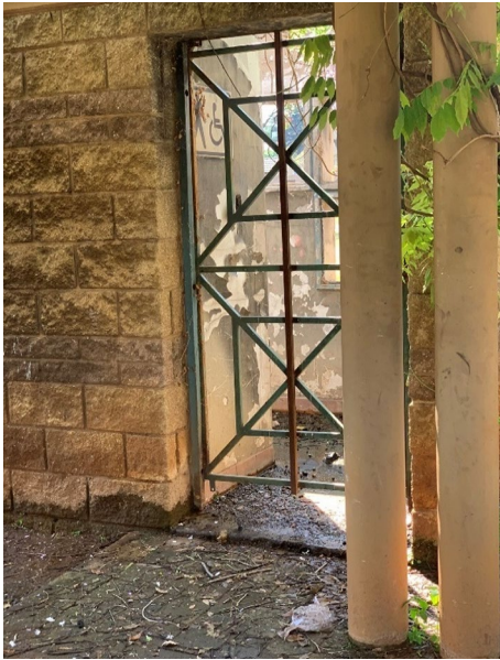
Fig. 7 Dilapidated restrooms at Venning Park
