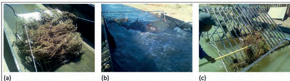
Figure 20. Debris blockage (a) during maintenance period (b) major debris build up after a 2-week interval (c) turbine removal and cleaning at 2-week interval
