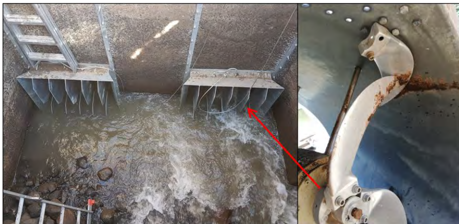
Fig. 8: Site 2 turbine damage due to large rocks
