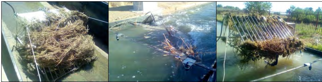
Fig. 6: Site 1 operational challenges due to debris
