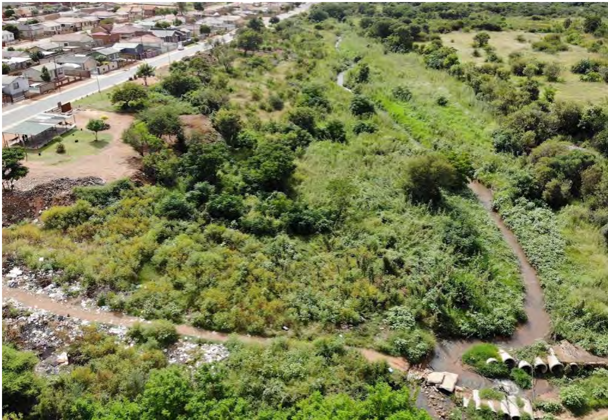
Photo plate 8: Oblique image of the damage to the bridge crossing the watercourse associated with community three
